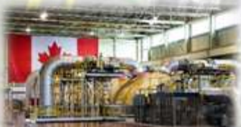
Pickering Nuclear Plant
